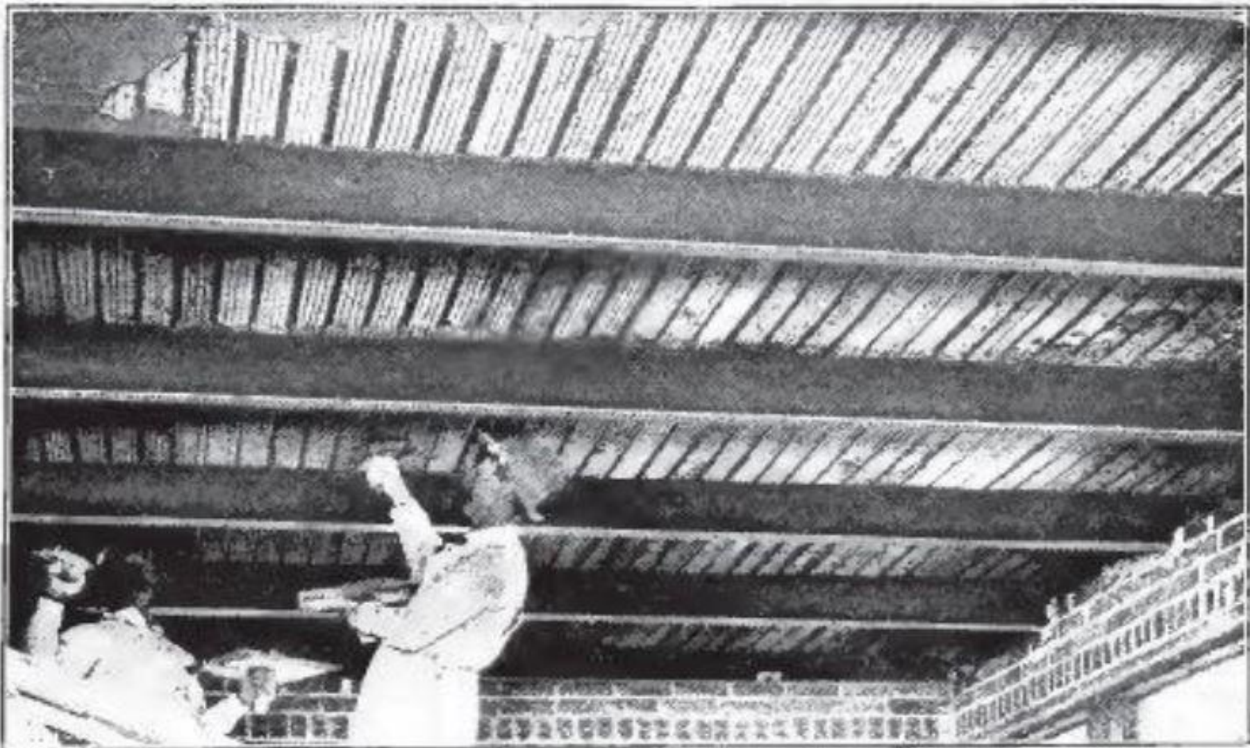
Plastering underside of Hy-Rib after being concreted above. View taken at Hotel Tuller, Detroit.
